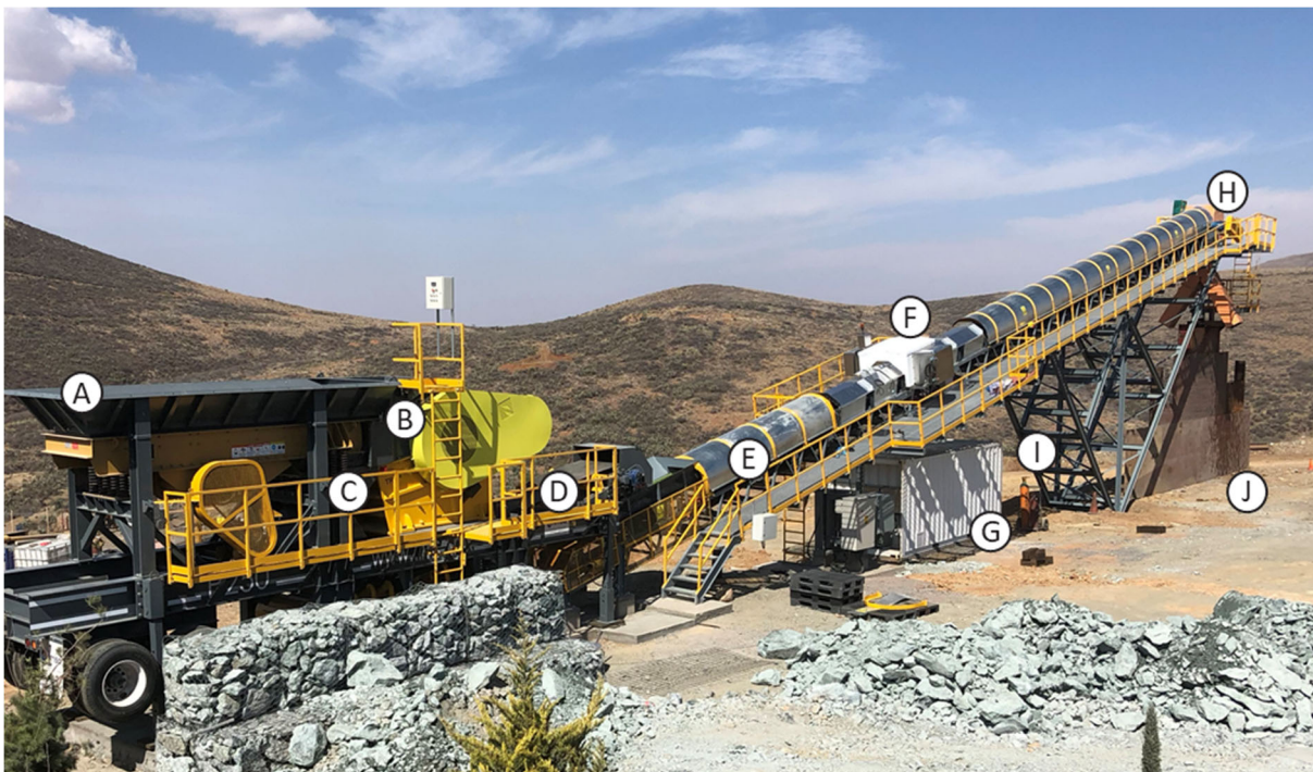
Figure 2 - Analyser installation before completing of the feed ramp, showing the hopper, crusher and feeder to the left, analyser and electronics container in the centre and diverter at the end of the conveyor.
